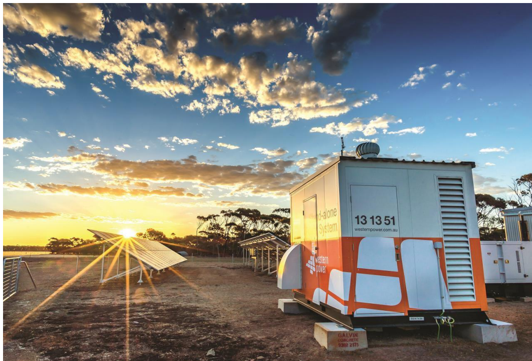
Figure 1: Stand-alone power system installed in West River in June 2016 as part of Western Power SPS pilot program.
