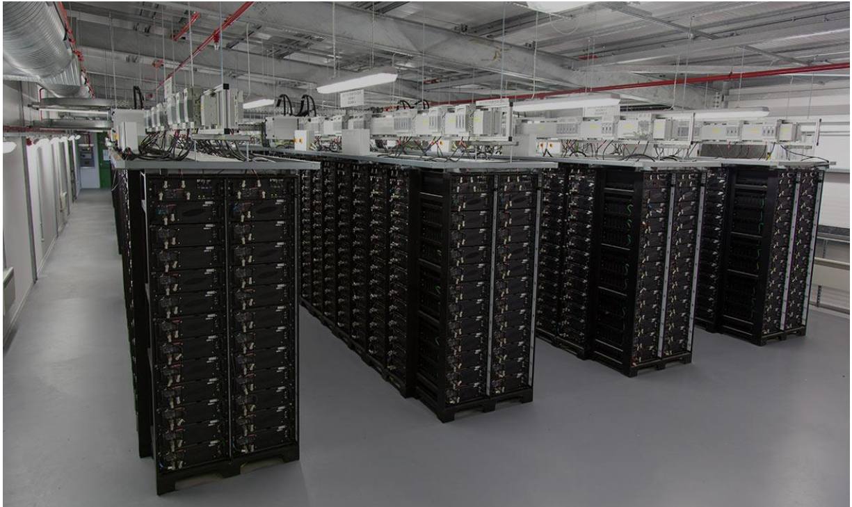
Distribution owned and operated 6 MW battery facility, UK Power Networks.
